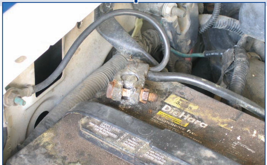
Figure 1: A loose negative battery cable explained the slow cranking, but wasn't the source of our problem.
